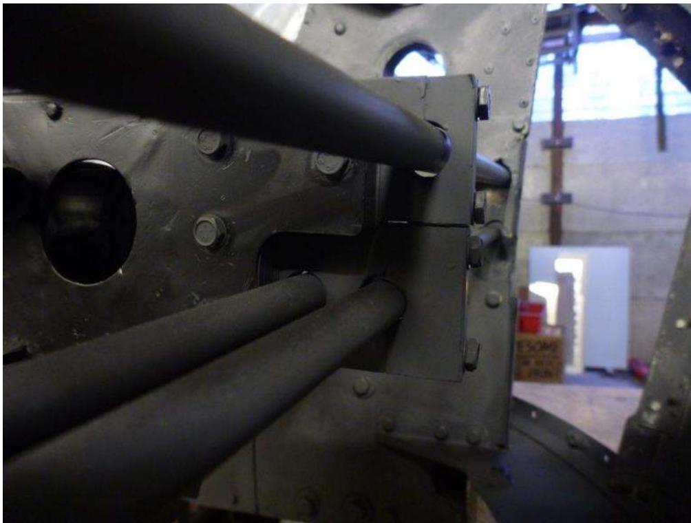
Control Rod Centre Support – This one is on the FN-5 as it is easier to photograph
